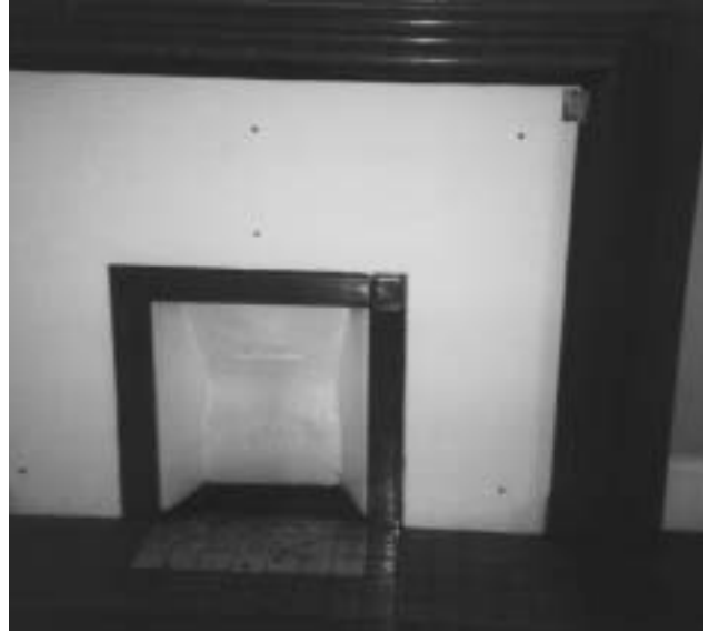
5e Painted AIB fire surround.
