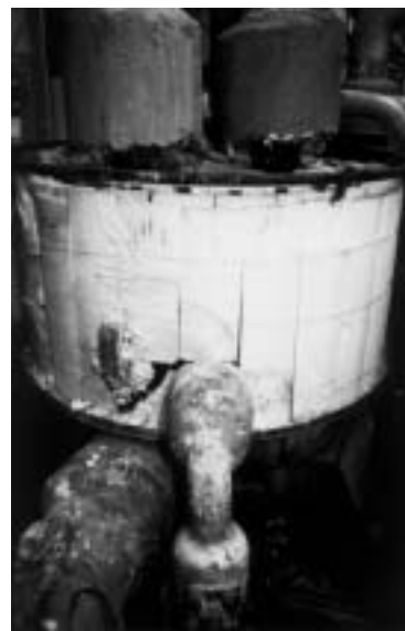
19a Asbestos-insulated vessel and supply pipes in a factory.
