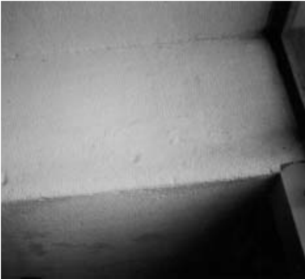
2a Cementitious sprayed chrysotile asbestos on a ceiling for decorative and fireproofing purposes, showing evidence of previous damage and repair.
