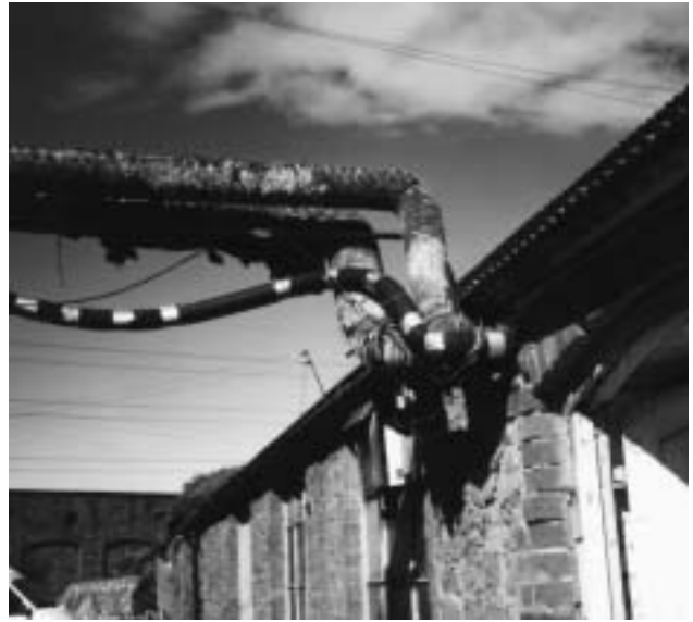
3h Badly degraded external asbestos-lagged pipe in an industrial plant, with asbestos rope wound around the bends.
