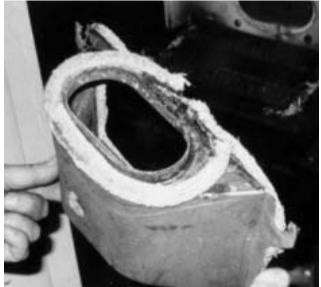
8d Asbestos rope seal in a domestic gas boiler.
