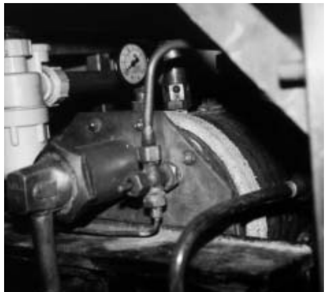
8a Example of asbestos tape on a domestic water heater.
