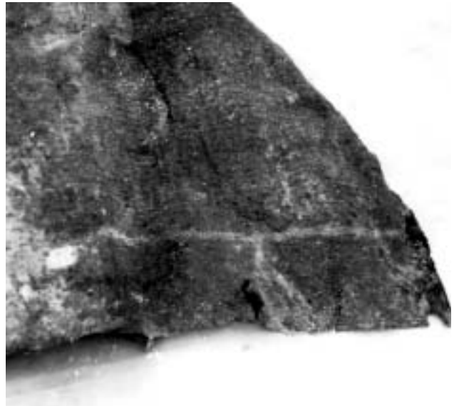
13a Weathered asbestos-containing roofing felt (less weathered material is black).
