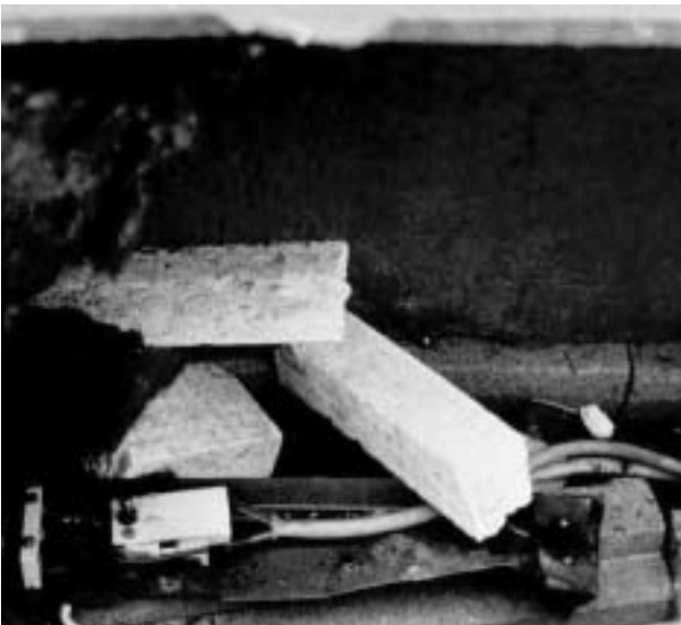
18b 'Caposil' insulation from inside an old electric storage radiator.
