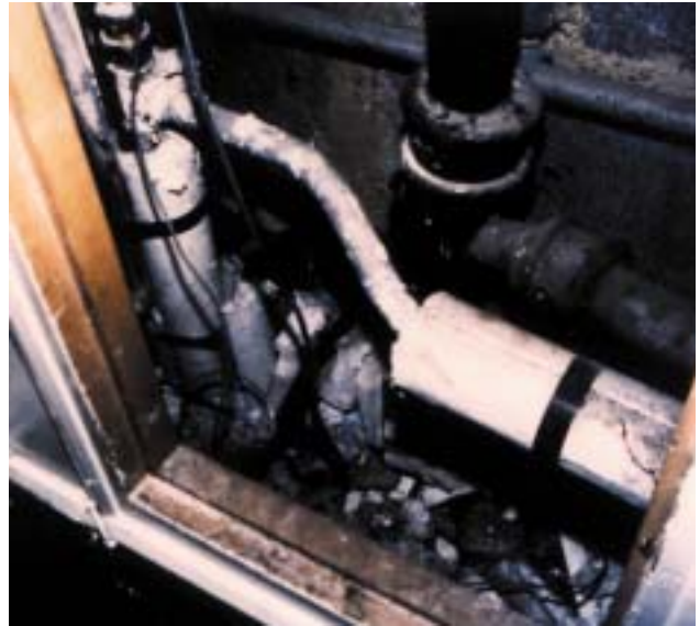
20a Asbestos debris in the bottom of a service riser.
