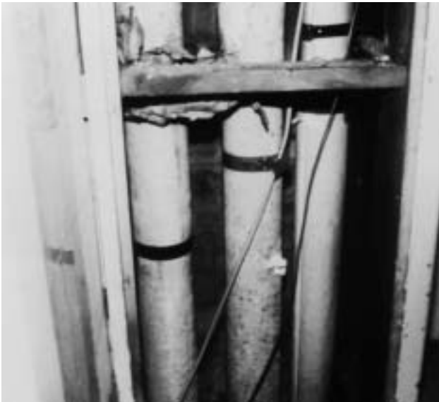
3c Asbestos pipe lagging in a service riser, with calico wrapping and straps.
