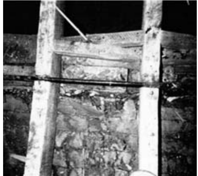
1b Loose insulation with paper cover degraded under a dance floor.
