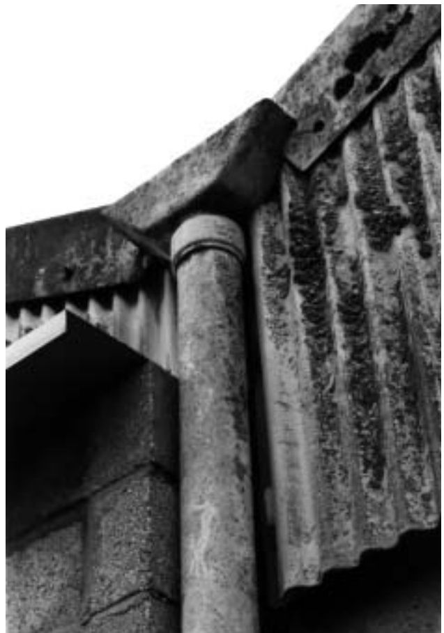
11d Asbestos cement downpipe, hopper and profile sheet.
