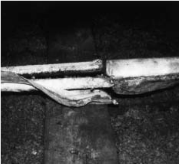
3b Asbestos-insulated water pipes in a loft, showing evidence of maintenance work damage, with detached pre-formed sections and calico wrapping.
