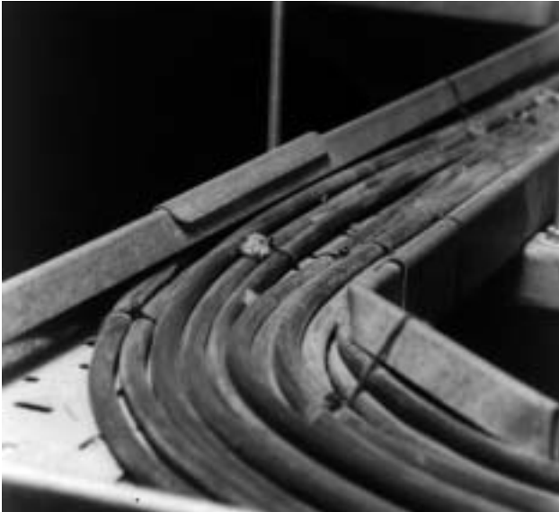
20c Fibrous debris in a cable tray.
