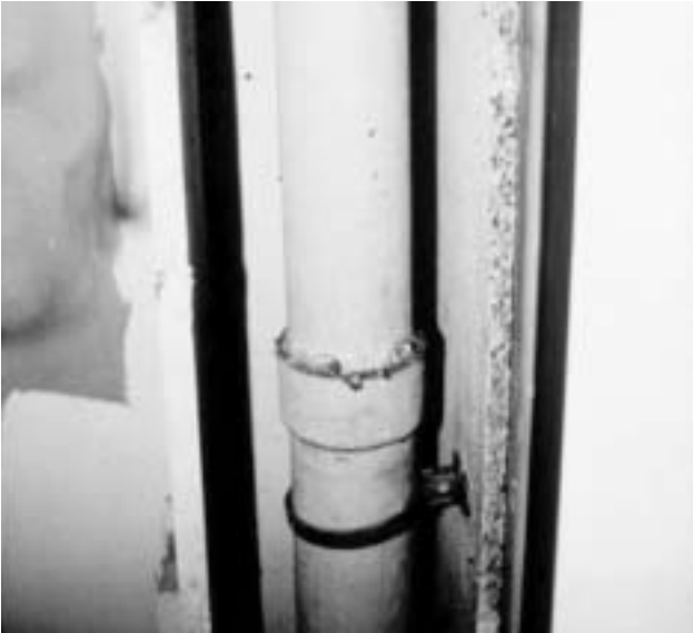
5d AIB around a service riser shaft (showing cut and uncut edges).
