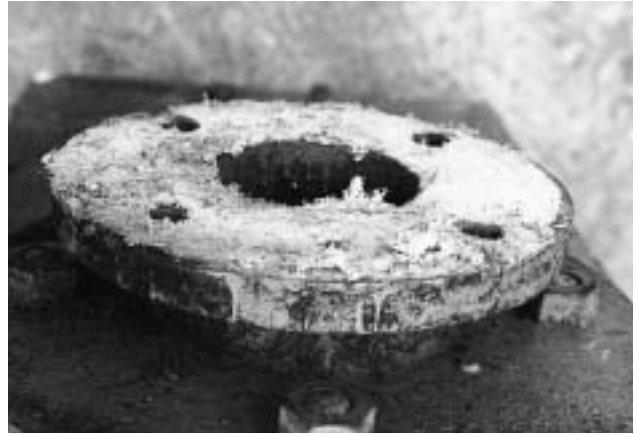
9c Gasket material adhering to a pipe flange.
