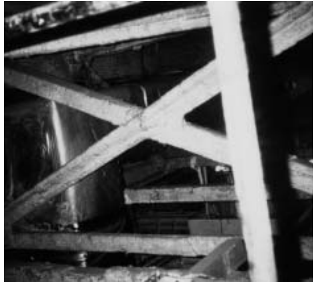
2c Sprayed amosite fireproofing on steel roof support beams in a return air plenum showing signs of damage and wear at the bottom caused by access for maintenance.
