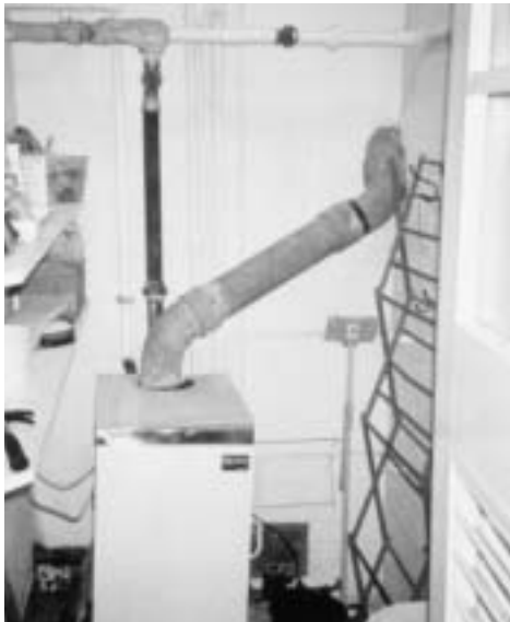
11b Asbestos cement flue from a domestic boiler.
