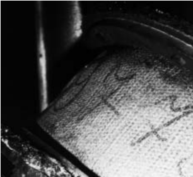
8b Asbestos gaiter between pipe flanges.
