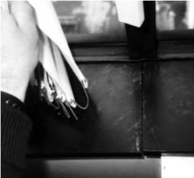
15b Asbestos-reinforced windowsill.
