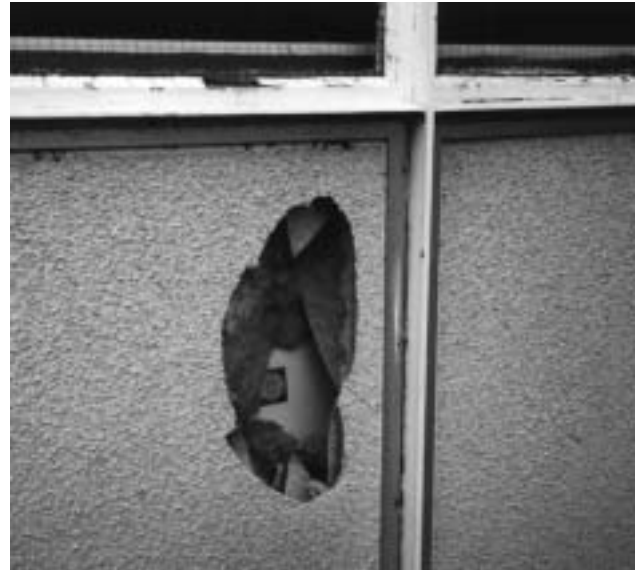
5a Typical use of AIB in system-built flats. The internal AIB panel is visible behind a broken flat sheet (possibly asbestos cement) with textured coating (possibly chrysotile asbestos-containing) with MMMF insulation in between.
