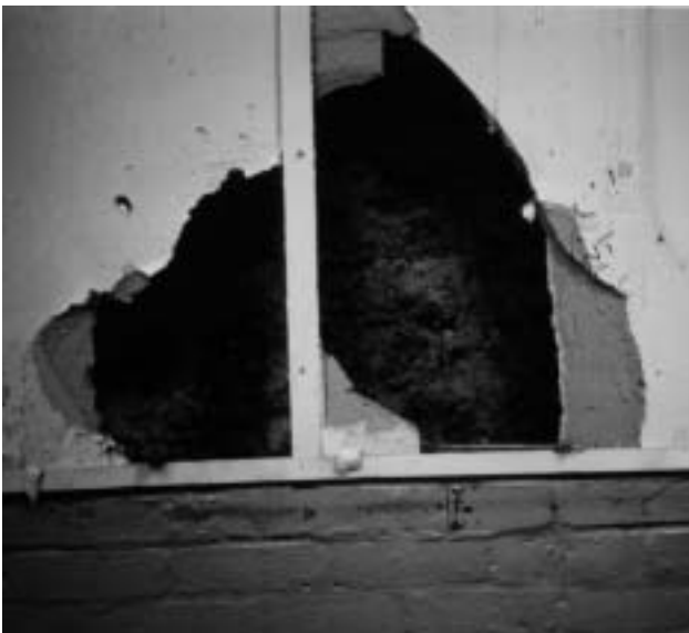
2f Sprayed crocidolite thermal insulation applied to external wall cladding and enclosed behind non-asbestos wallboard.
