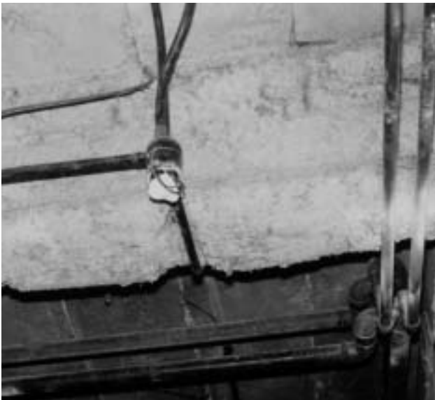
2b Poorly tamped sprayed chrysotile fireproofing on a structural steel beam holding up a concrete floor showing some overspray onto the concrete and damage by electrical work.
