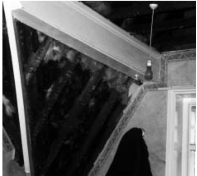
21a Glasswool insulation usually has a distinctive yellow colour, even after many years of gathering dust in lofts and roof spaces. A black layer of asbestos-containing roofing felt is, however, visible where the insulation has been removed and the wooden roof purling is encased in AIB. Rockwool and slagwool are also widely used and their darker brownish or grey colour may possibly be confused with amosite, although the texture and fibre size is very different from asbestos. These wools may occur in blanket form, pre-formed bats and blown as loose insulation in cavities. MMMF textiles have a vitreous shiny appearance (see 9a) compared to asbestos textiles.
