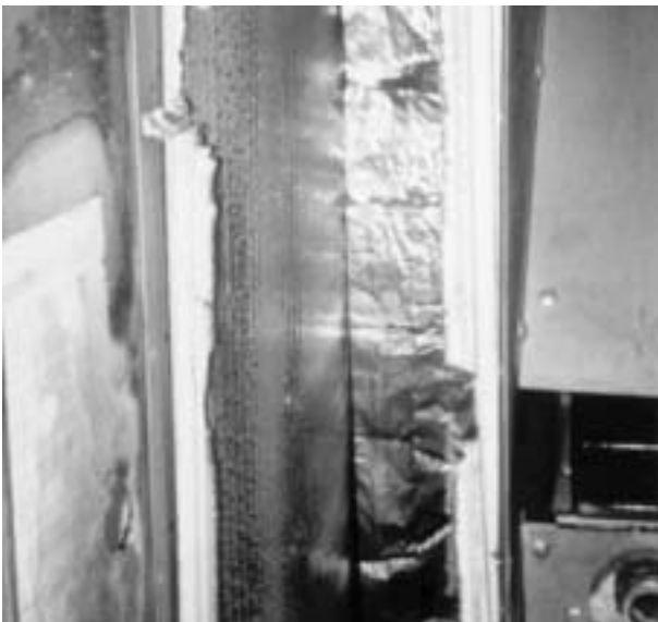
7b Foil-backed asbestos cardboard insulation inside a warm air heater.
