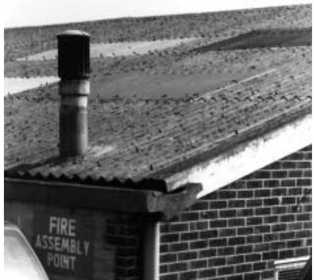
11c Asbestos cement external flue, rain water gutter and profile roofing sheet.
