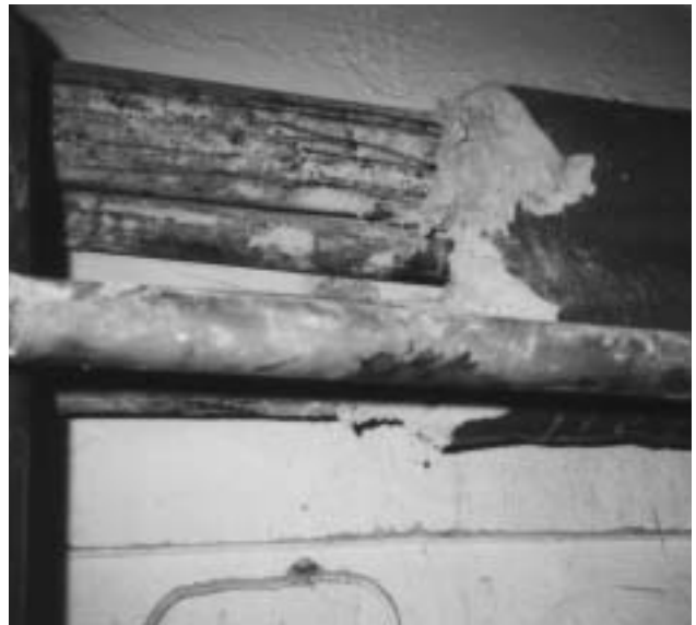
3i Example of hand-applied 'hard set' insulation, partially removed from a pipe.
