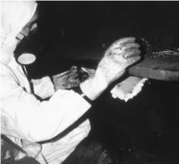
4a Removal of a piece of low density millboard from an electrical cable box.
