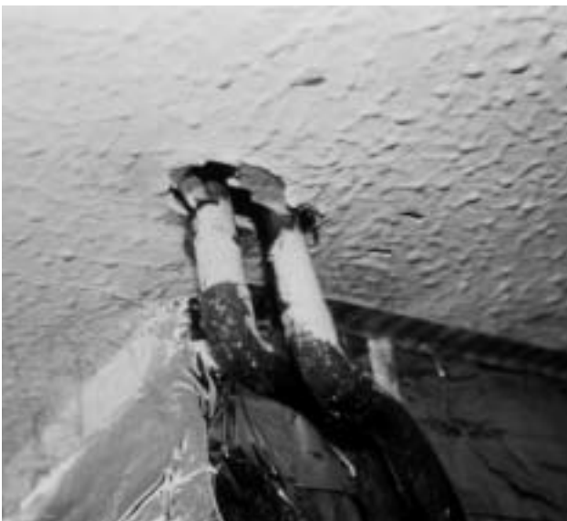
12a Example of painted chrysotile textured coating on a ceiling.
