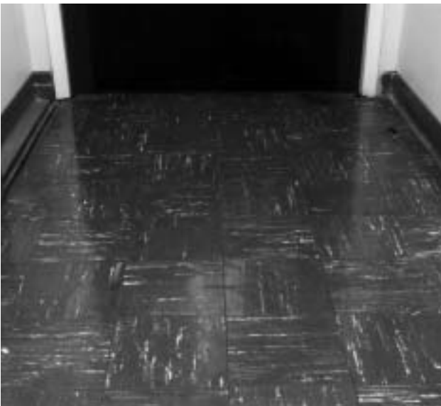
14a Asbestos-containing vinyl floor tiles.
