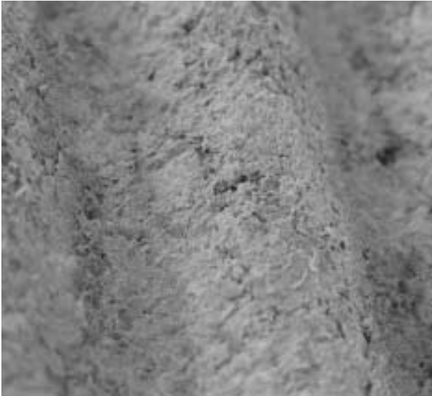
2e Close-up of the surface of sprayed amosite insulation (~40 mm thick) on the underside of an asbestos cement roof.
